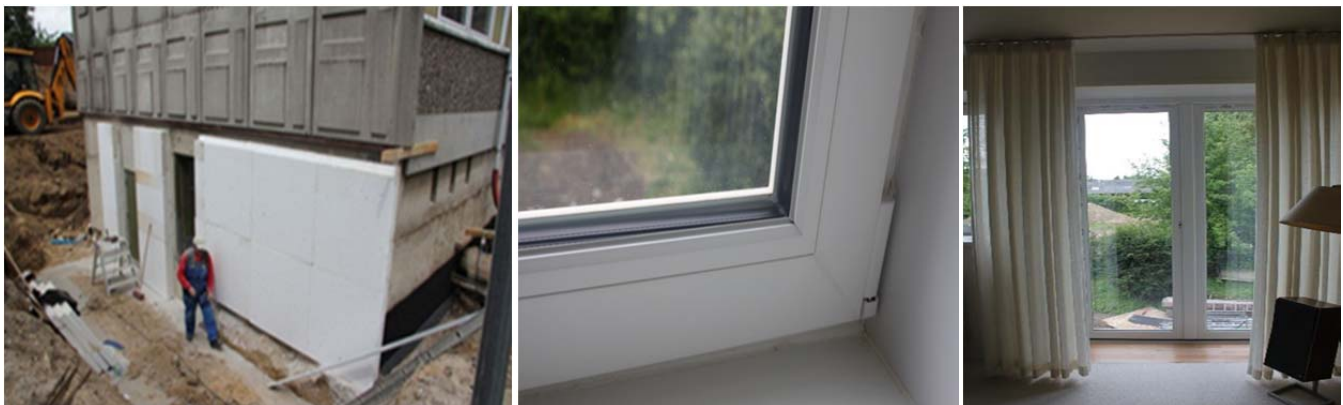
Fig. 2. (a) The external insulation (EPS) of the basement walls; (b) Lower corner of a plastic triple-glazed low energy window; (c) New balcony doors – plastic with energy-efficient glazing.
