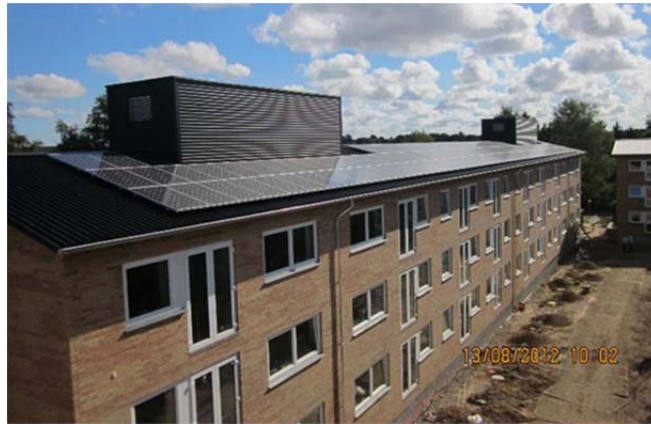
Fig. 4. The 33 kWp south-facing PV system and the coverings for the new mechanical ventilation systems located above each stairway.
