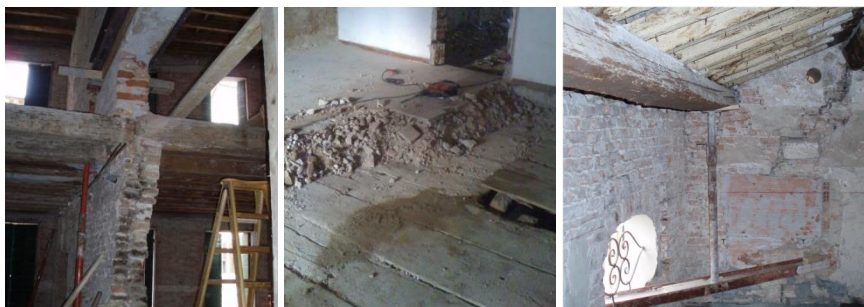
Fig. 2 Building envelope before renovation: a) crooked walls; b) demolished partition walls left and used as a substrate; c) beam support in the perimeter wall.
