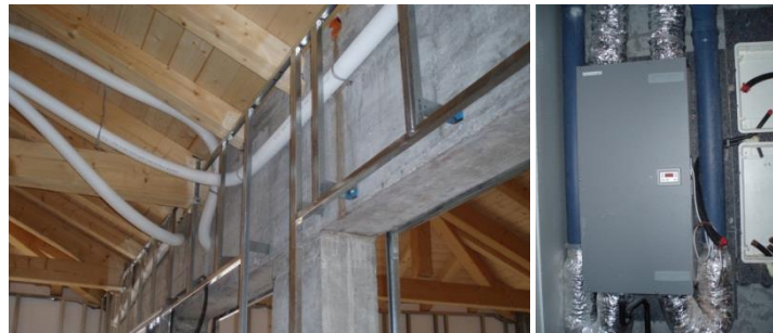
Fig. 5 Mechanical ventilation system.
